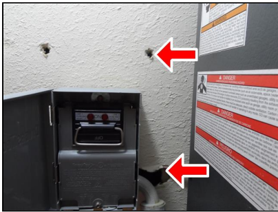
Air handler closet
