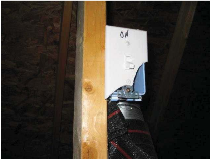
Broken light switch cover at the attic
