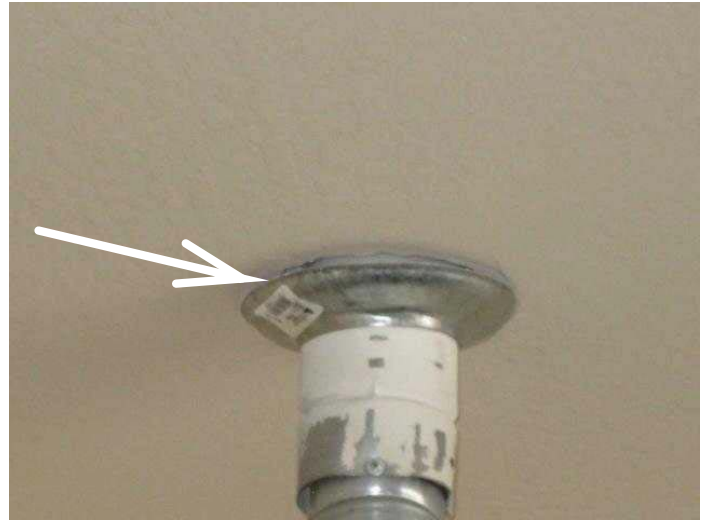
Water heater flue pipe fire ring not properly secured at the garage ceiling
