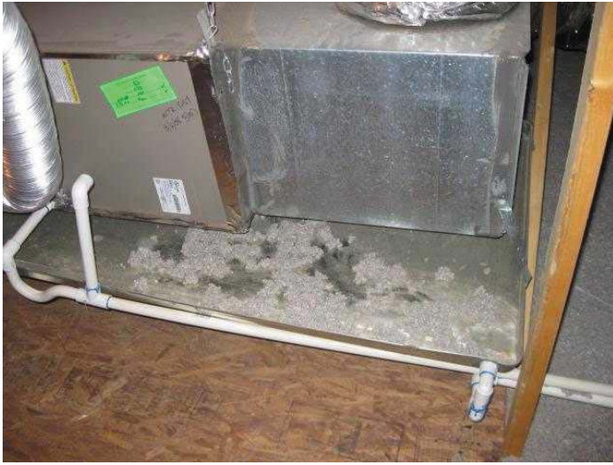
Insulation in A/C condensation drain pan at the attic
