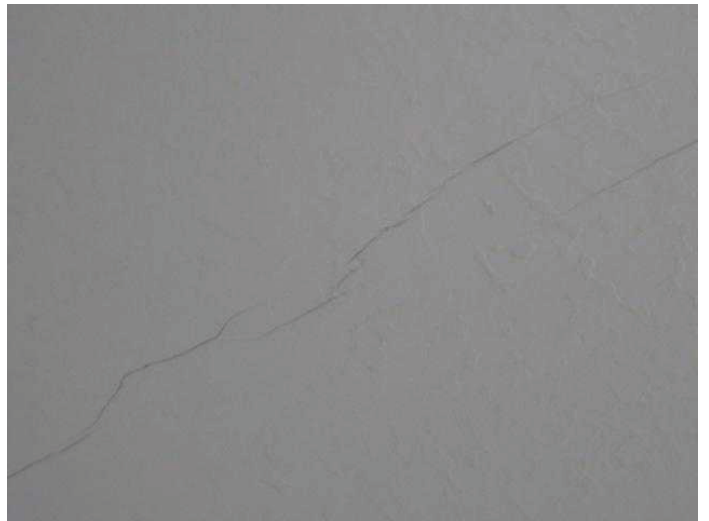
Cracking at garage ceiling
