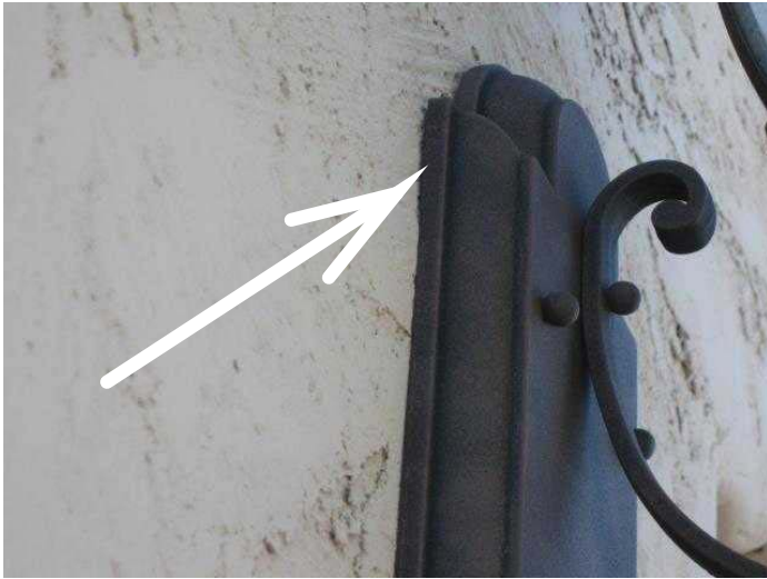
Caulk around exterior light fixtures
