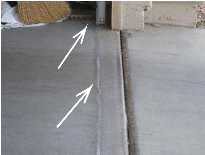
Evidence of water entering garage under door
