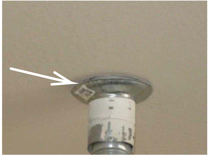
Water heater flue pipe fire ring not properly secured at the garage ceiling
