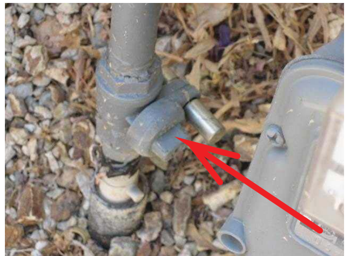
Gas off - Meter locked
