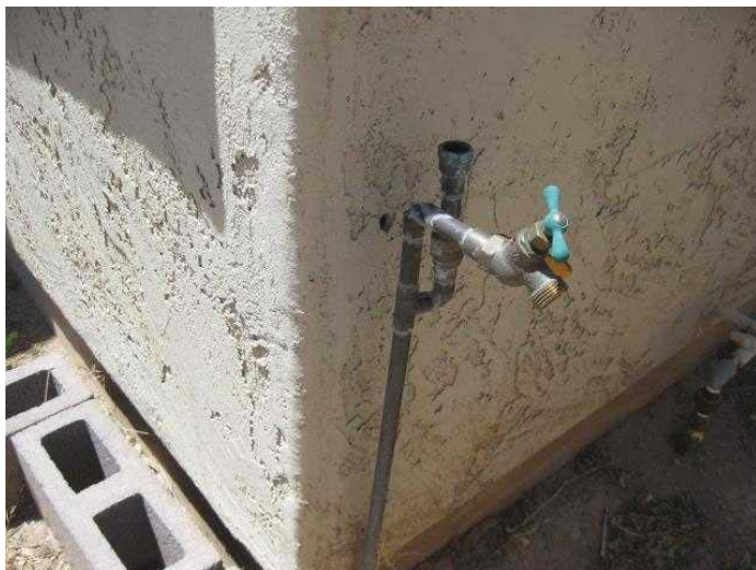
Hose bib piping not secured to the wall
