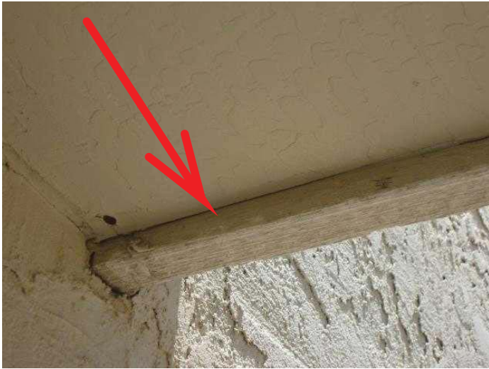
Seal gaps at patio ceiling
