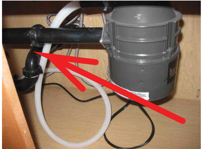
No sanitary loop at dishwasher drain
