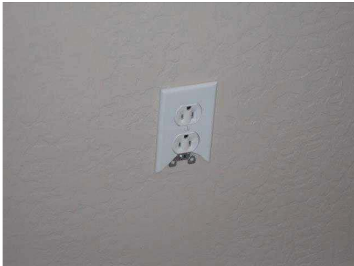
Damaged outlet cover at the loft
