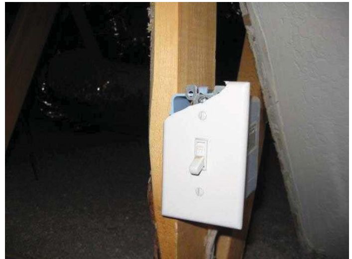
Damaged switch cover at the attic
