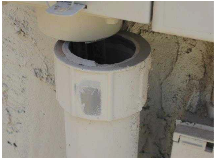
Damaged electrical service entrance conduit
